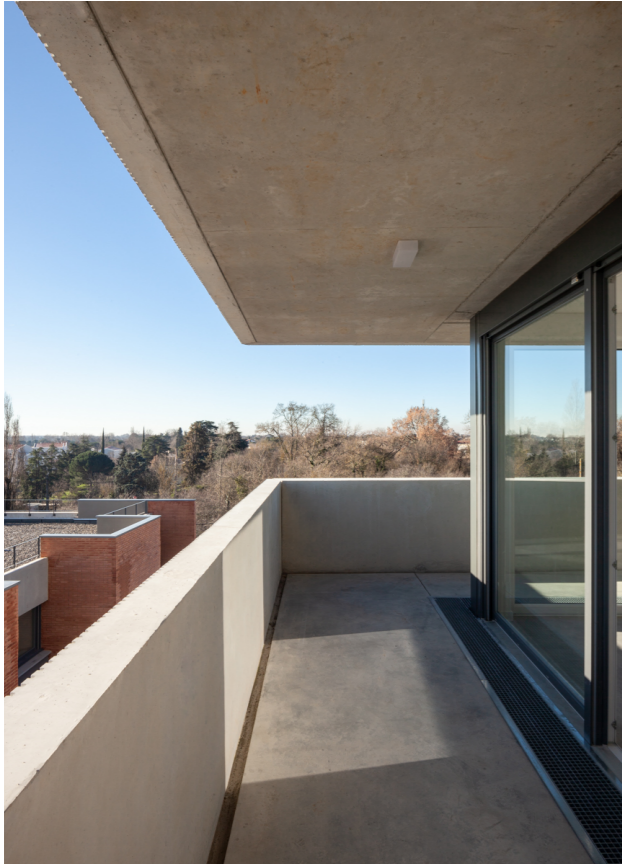
Balcon des étages courants du grand bâtiment. Balcony of the typical floors of the large building.
